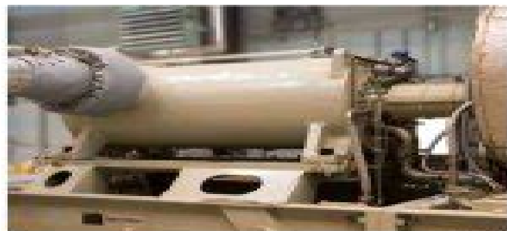
C61 Gas Compressor
