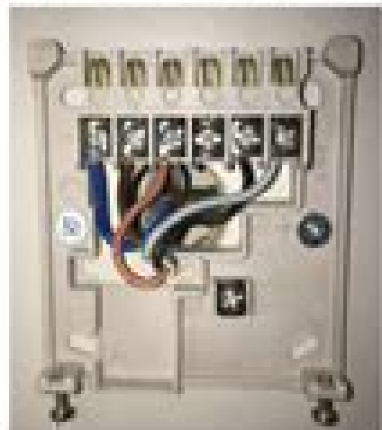
Back plate wiring
